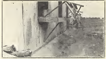
FIG. 9. Compania Agricola de Ulua, Zapote Camp, Republic of Honduras. Concrete gutters for slops at the rear of the kitchens of the laborers' houses. Waste water from pumps goes into these same gutters.
